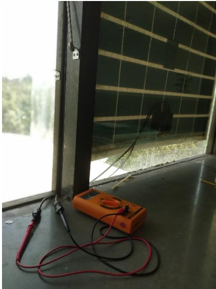
Connection between multimeter and panel for measurement of readings
